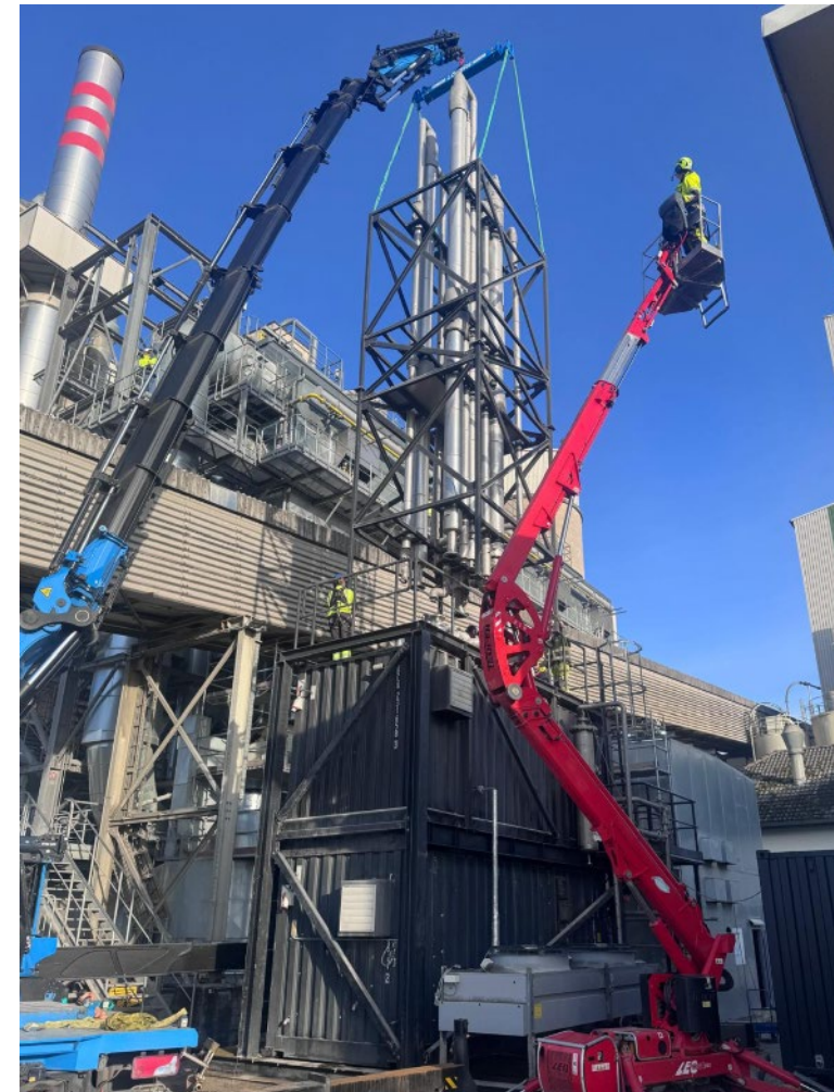
Ongoing: Demonstration at Dyckerhoff Cement plant in Germany with liquefaction - 2026
